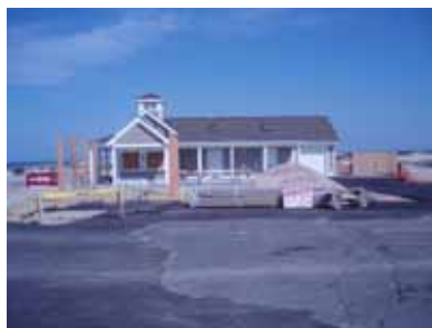
The bathhouse is almost completely finished. Stairs are in. Cupola is in.
