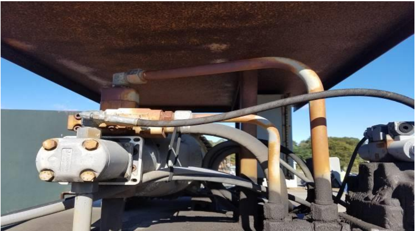
Compactor Units at Transfer Station
