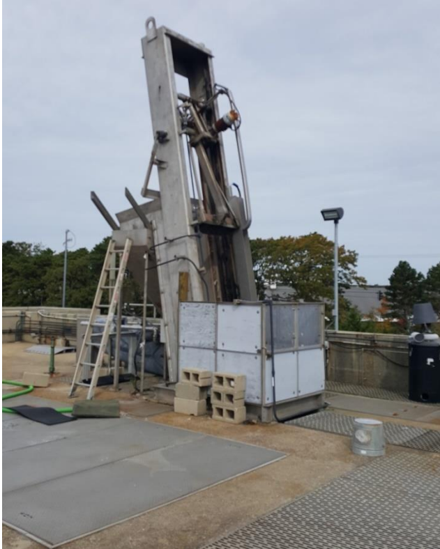
Mechanical Bar Screen
