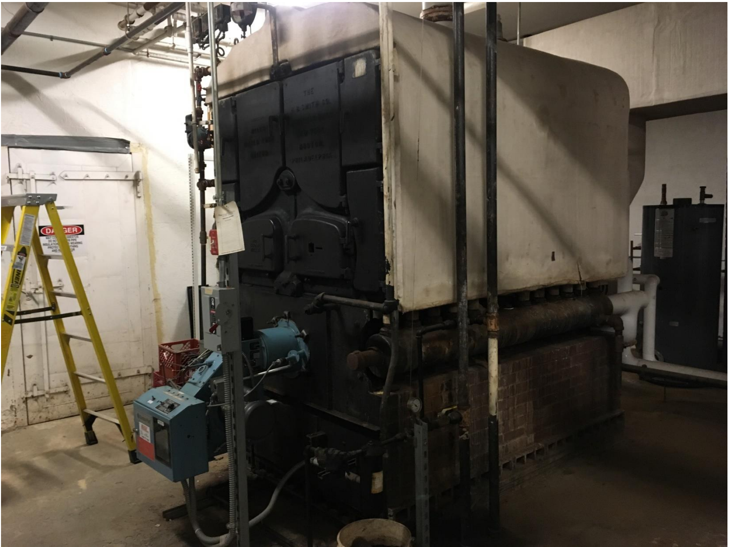
Barnstable West Barnstable Boiler
