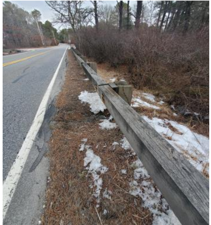
Runoff from Santuit Newtown Road under the guardrail to Lovells Pond. Taken February 2021.
