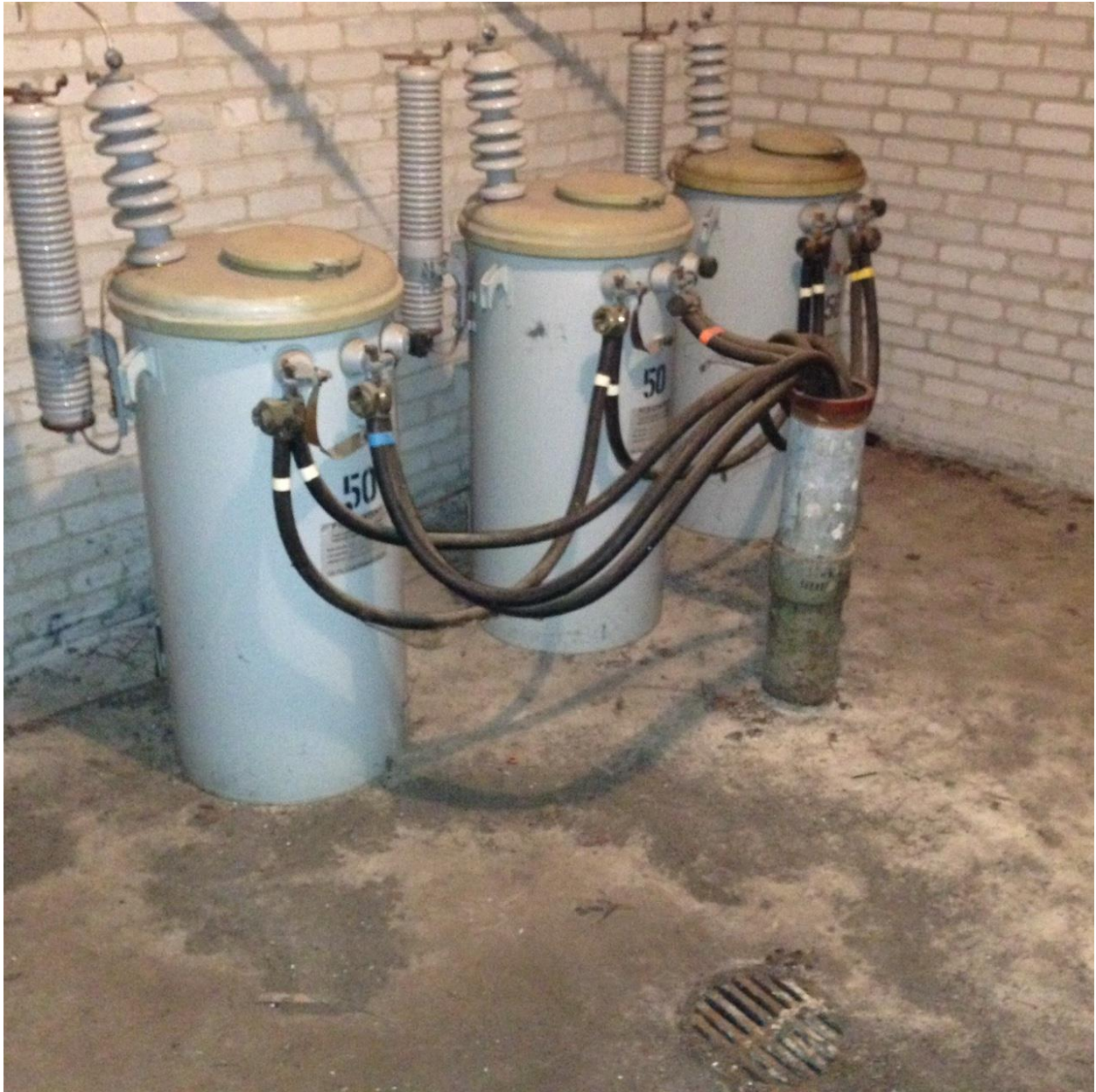
Typical Underground Transformer Array
