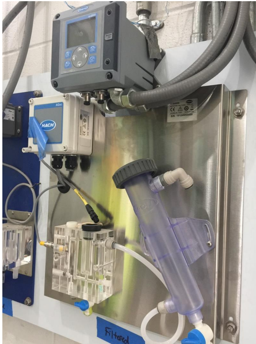
Water Treatment Equipment
