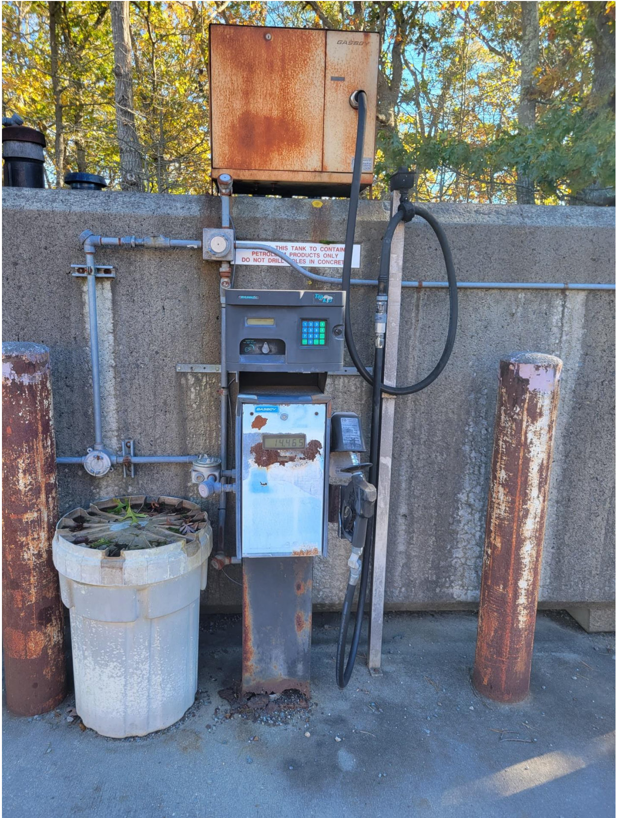
Facilities Fuel Pump
