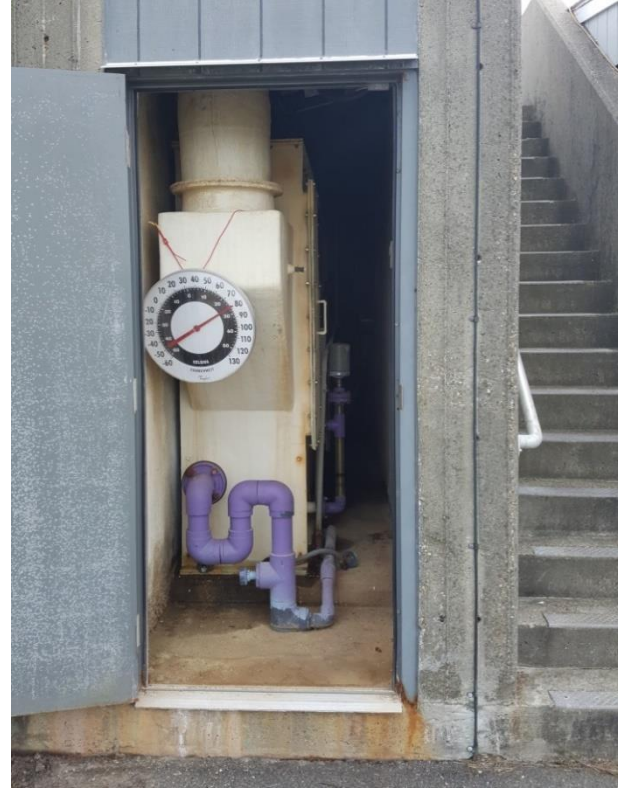
Odor Control System Access
