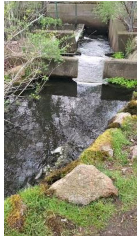
Worn steps and pools along fish ladder.
