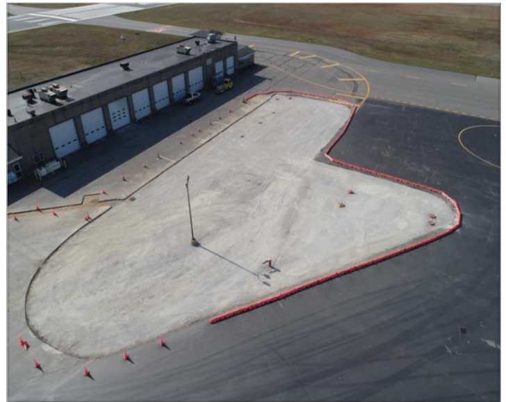
Photo shows excavated PFAS impacted soils removed and ready for asphalt cap as a permanent solution for mitigation.
