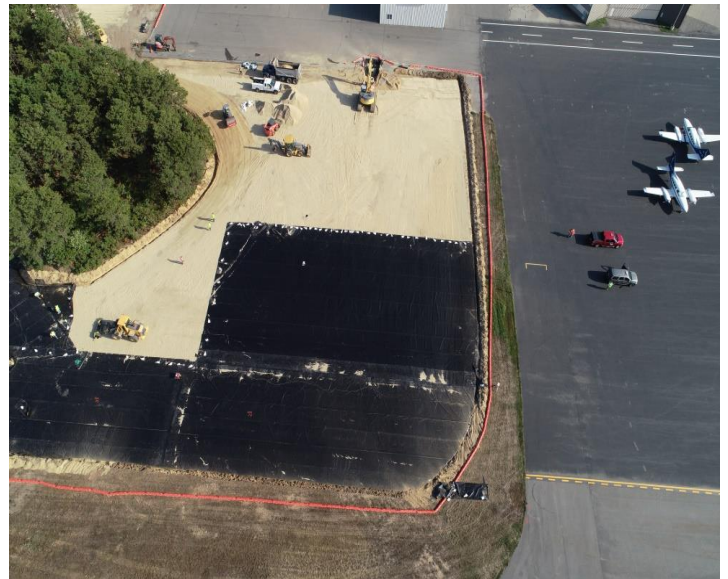
Photo shows excavated PFAS impacted soils removed and installation of a poly-fiber cap as a permanent solution for mitigation.
