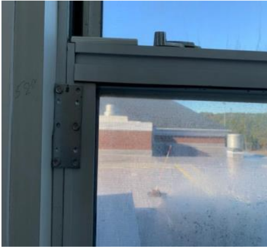
School Windows Needing Replacement
