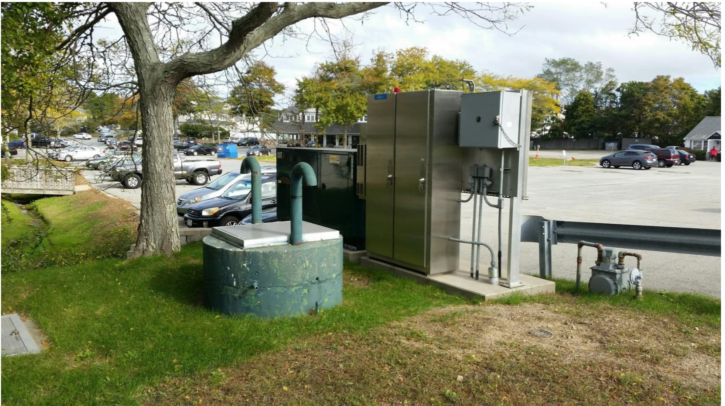
Existing 720 Main Street Pump Station
