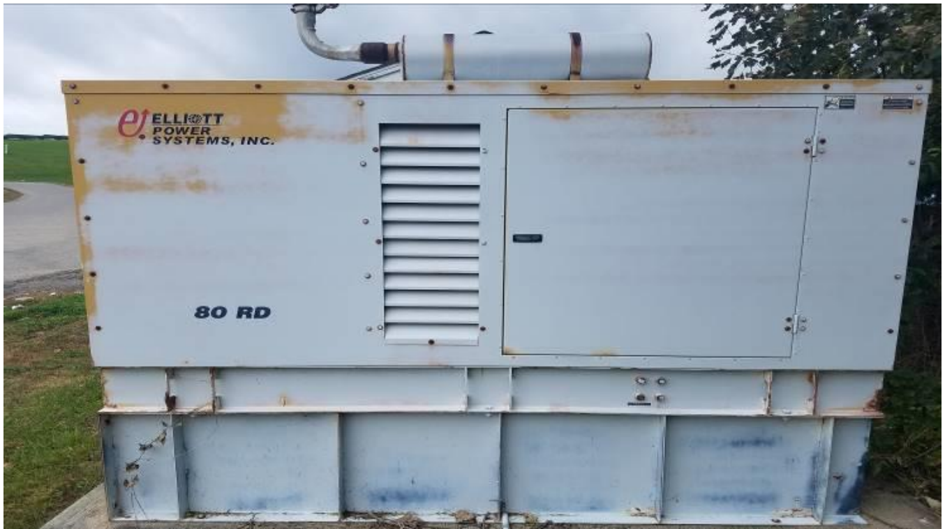
Generator used for the trash and recycling compactors is over 15 years old
