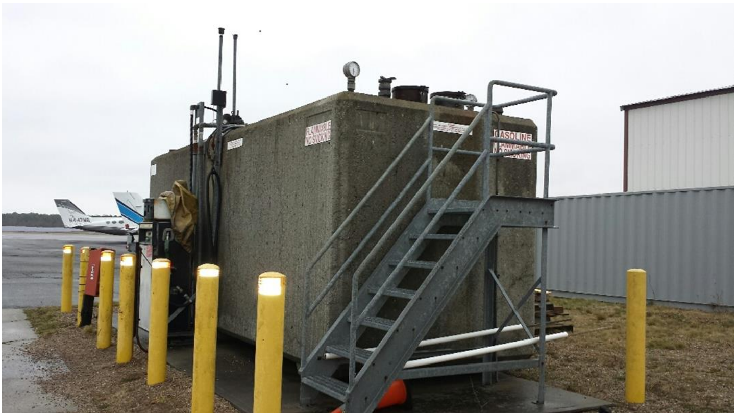
Circa 1997 Mo-Gas and Diesel Fuel Con-Vault, Gas Boy & Alarm
