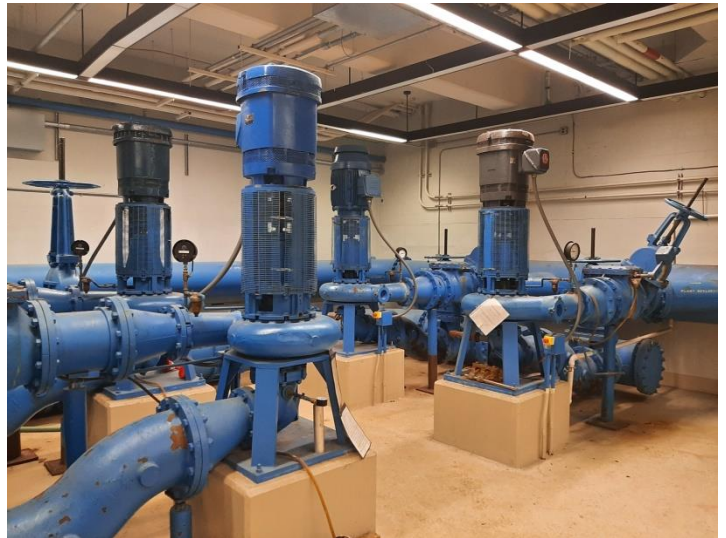
WPCD Effluent Pumps, installed in 1980
