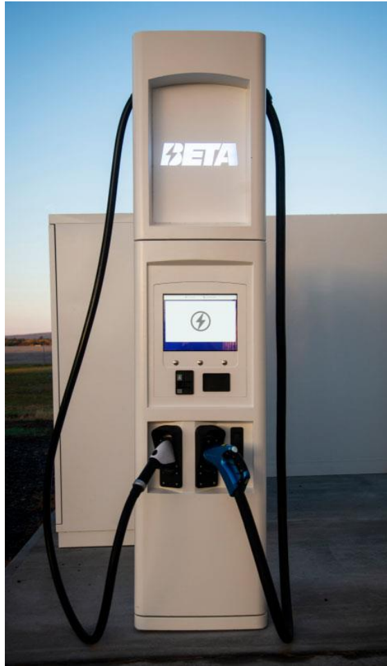
Electric Charging Station
