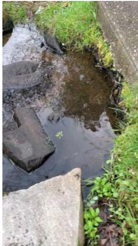
Water flow from pond under the sidewalk caused undermining.
