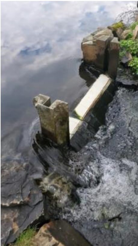
Stone damage and missing stones around the water control structure.
