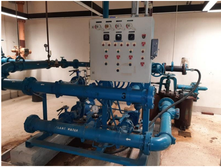
Plant water system, installed in 1980
