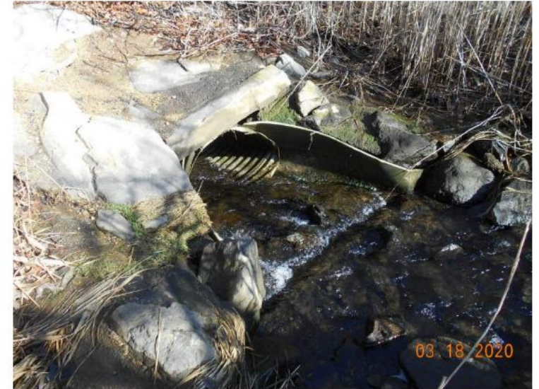
Photograph #3 – View of the existing culvert to the east of Commerce Road.
