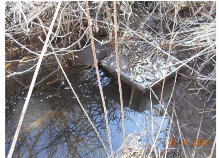
Photograph #4 – View of the existing culvert to the west of Commerce Road.
