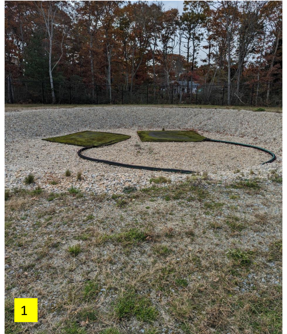
View south of existing backwash basin to be filled in for Straightway new facility stormwater management system
