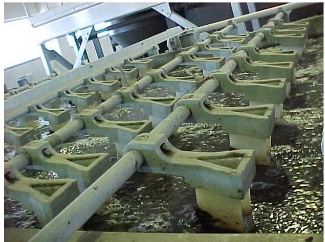
Waste Water Plant Activated Sludge Process
