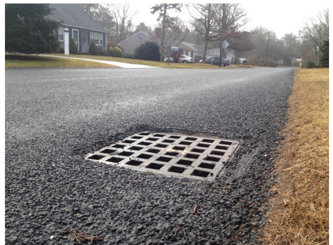
Storm Drainage System
